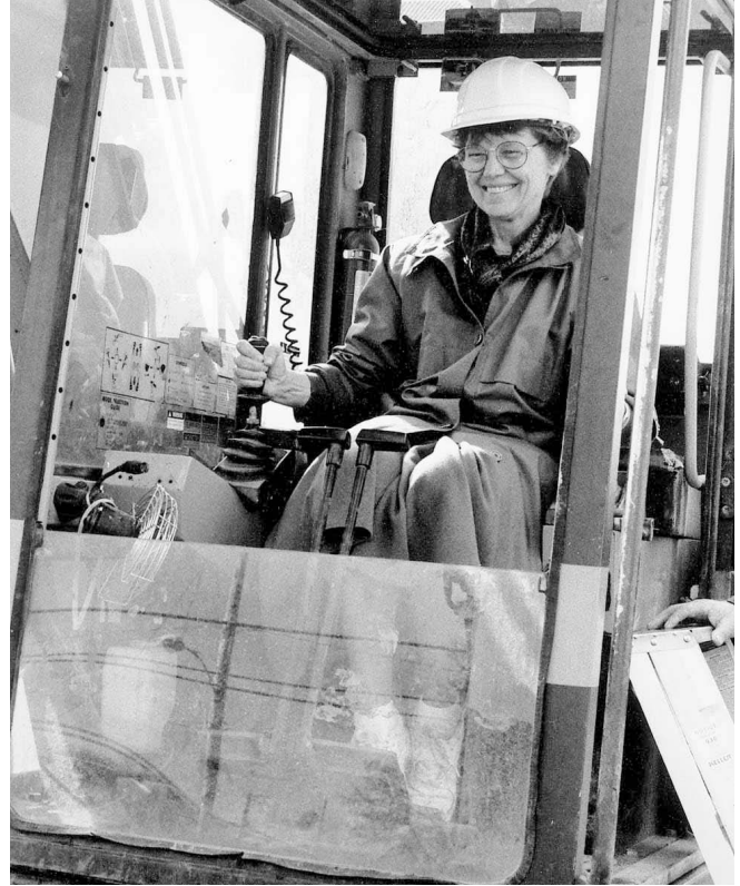
Vivian Bull can add heavy equipment operator to her resumé. She’s driven backhoes and trackhoes, breaking ground, breaking walls and tearing down fences. Here, she breaks ground for the Ad and Joan Rutschman Field House.
