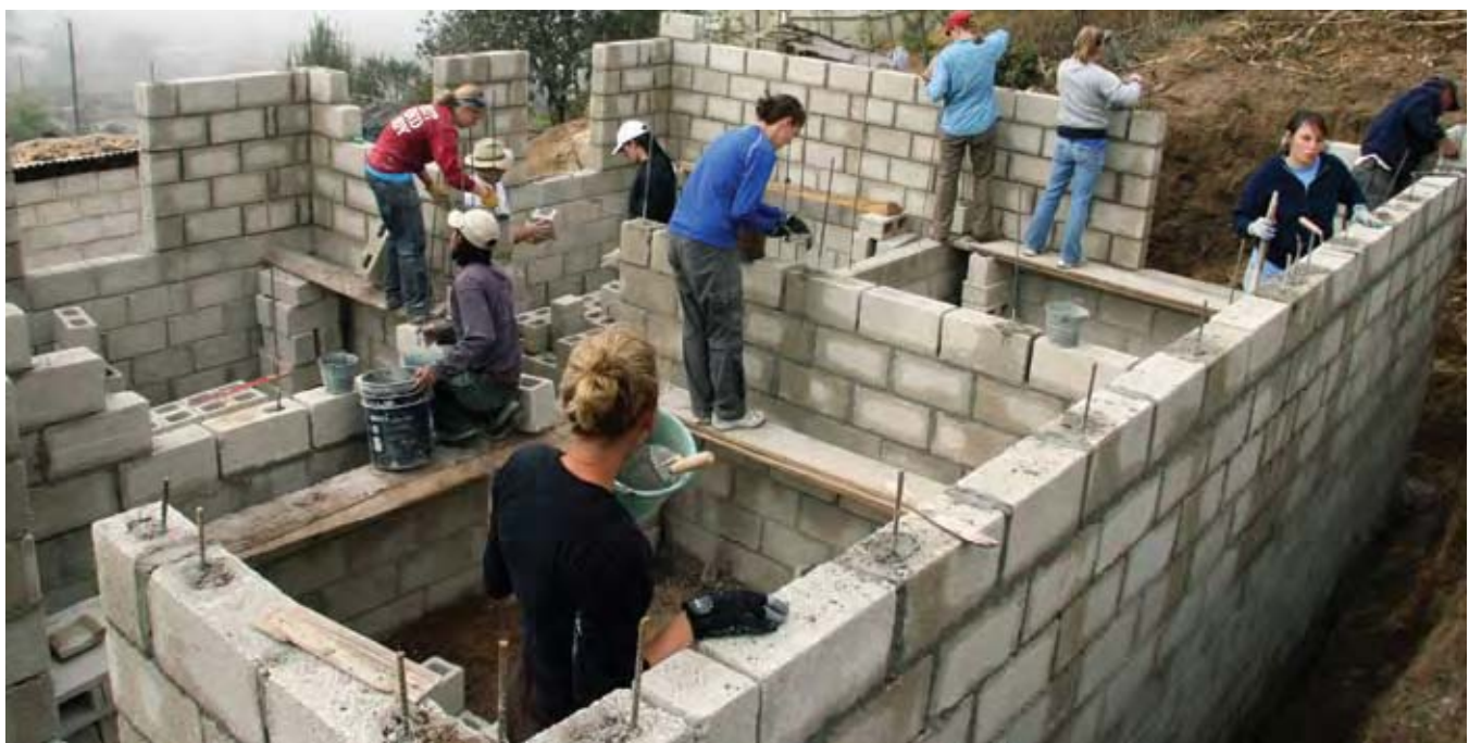
Linfield students and McMinnville community members worked together on four Habitat for Humanity houses during a January trip to Guatemala. Linfield students plan to return to Guatemala in March for an alternative spring break project. This home, located on a rural site in the steep hills outside Quetzaltenango, is nearly ready for a roof.
